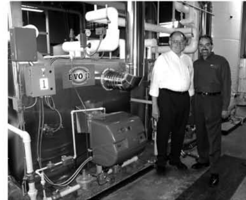
A happy customer! Bodo Langusch and Stucky show off the new EVO II units installed at Metropolitan.
